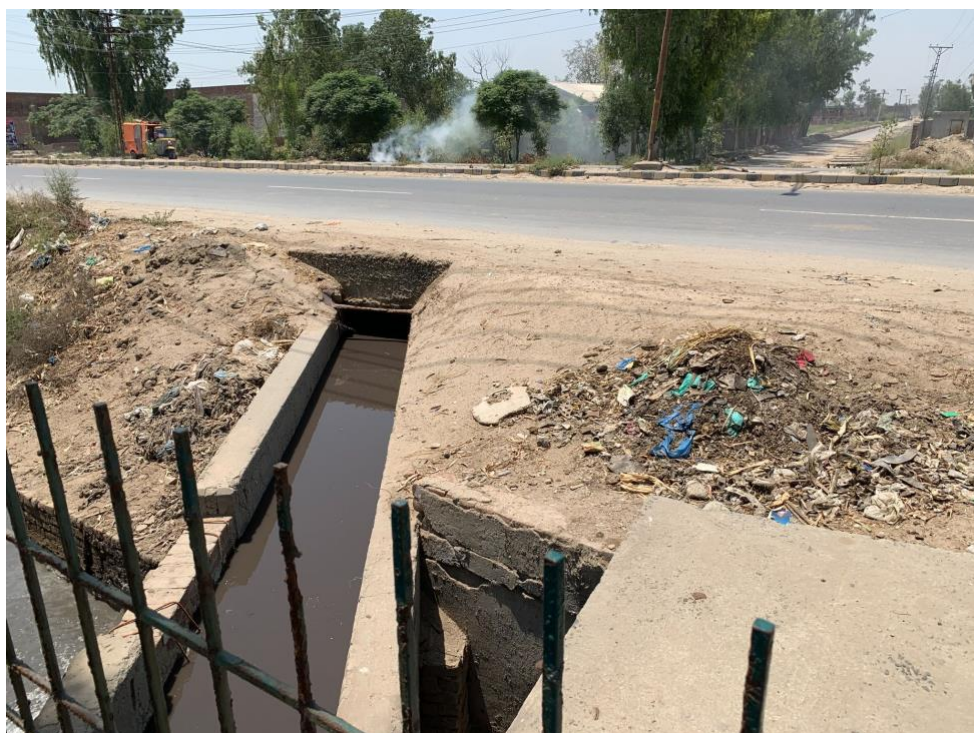
Figure 14: Dumped garbage and waste burning observed outside Kasur CEPTP
