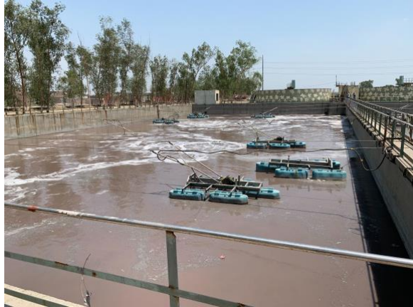
Figure 11: Two large Aeration ponds
