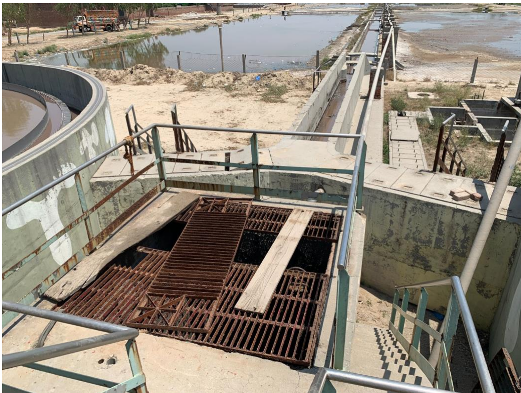
Figure 15: Water tank at CEPTP where accident occurred; remains poorly maintained
